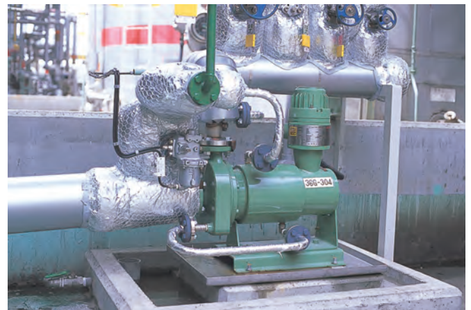
High melting point type pump in a chemical plant.
