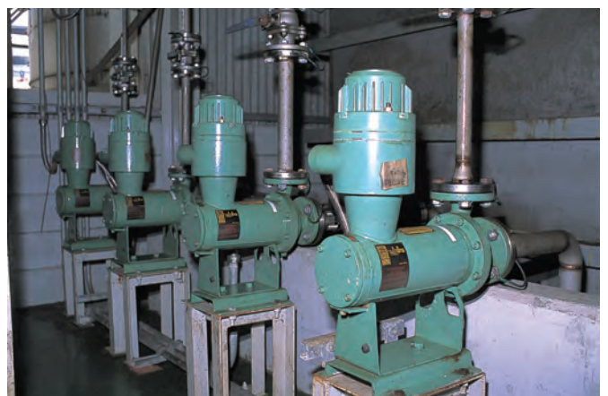
Basic type pumps in a chemical plant.
