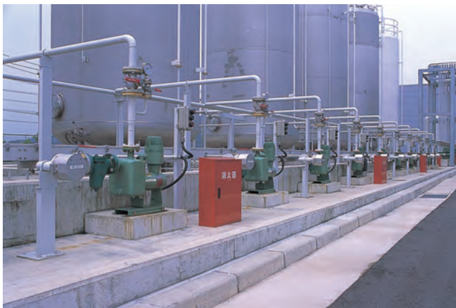
Self-priming type pumps in a paint manufacturing plant.
