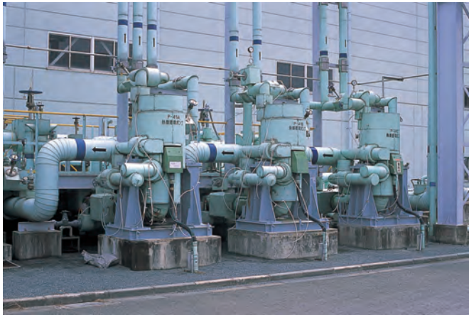
Reverse circulation type pumps for pumping LNG as Cooling medium. (Vertical type, Motor output 75kw)
