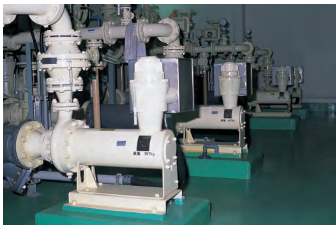
Basic type pumps in a water treatment plant. (Titanium casing & impeller)
